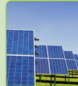
Solar energy generation
